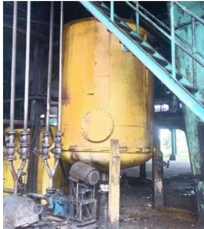
Gambar 3. 17 Sand Trap Tank
