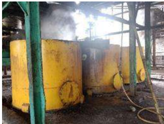
Gambar 3. 19 Crude Oil Tank
