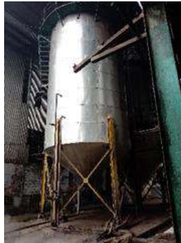
Gambar 3. 20 Continuous Settling Tank
