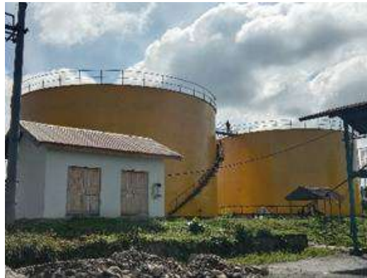
Gambar 3. 24 Tangki Timbun (Storage Tank)
