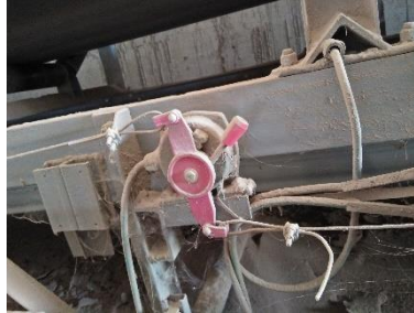
Gambar 3.10 Sensor Rope Switch
