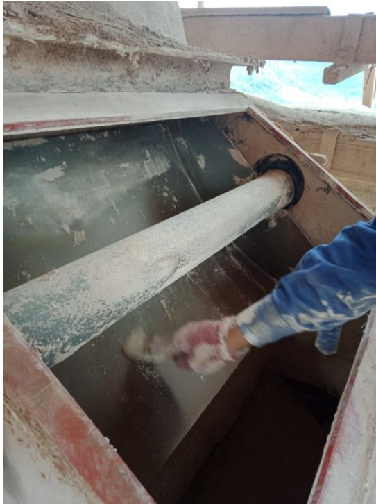
LAMPIRAN 13 (Flow Meter)
